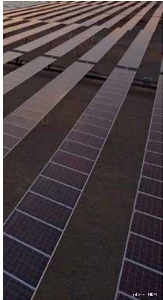
Solar PV panels
